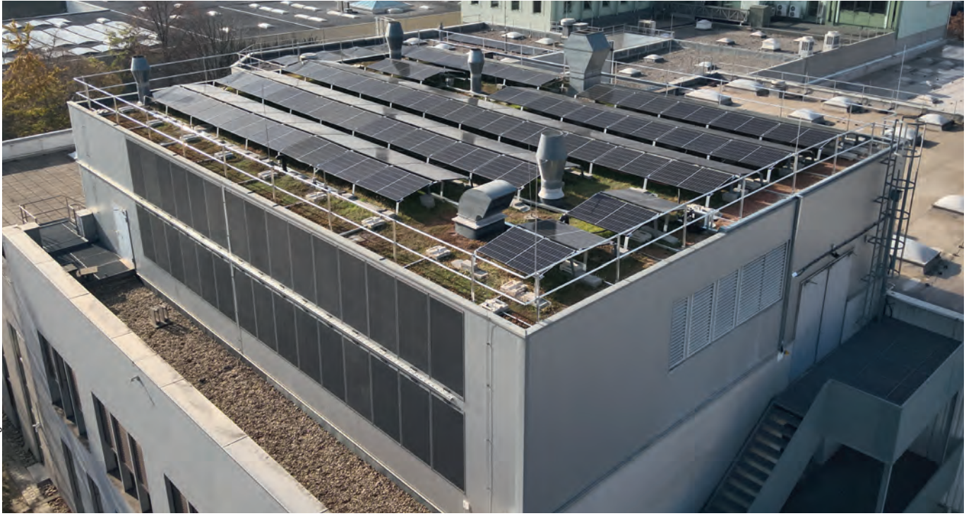
Photovoltaikanlage © Schwabe Austria
